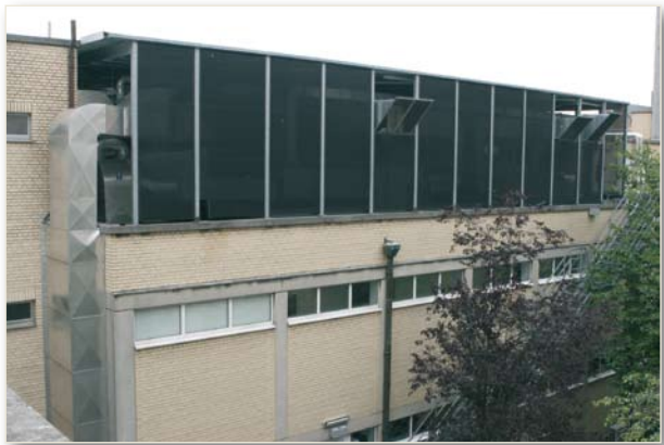
The L3-building with elaborate technical machinery on the rooftop.
